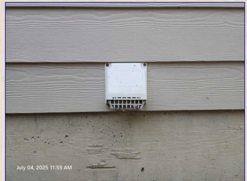
The Dryer Vent
