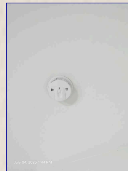
The smoke/CO alarm operating.
