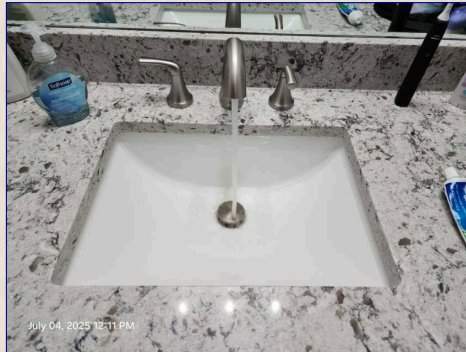
Sink faucet operating
