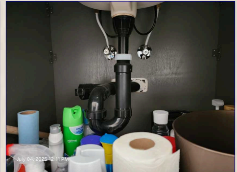
The bathroom plumbing view.
