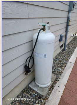
The main gas shutoff
