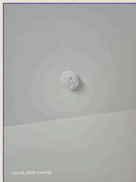
The smoke/CO alarm operating.
