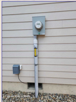
The electrical service entrance
