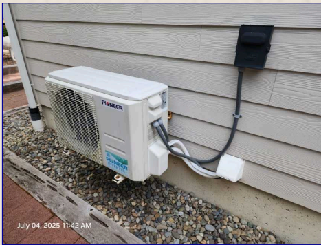
The air conditioner compressor/condenser area.
