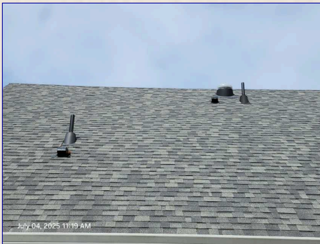
The Plumbing and Bathroom Vent(s)
