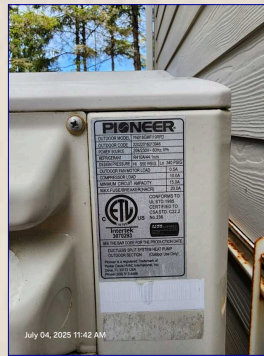
The air conditioner compressor/condenser data plate.
