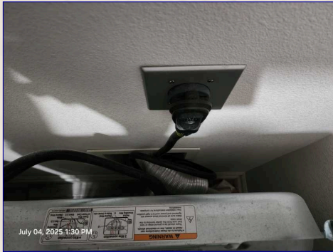
The dryer hook-up view
