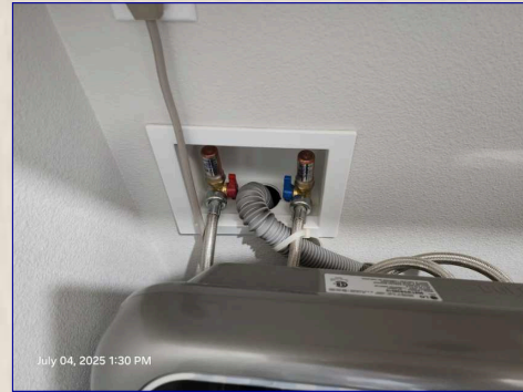
Laundry, washer hook-up view
