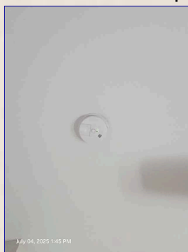
The smoke/CO alarm operating.
