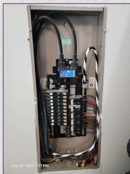
The main electrical service panel
