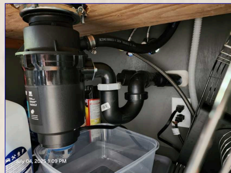
Kitchen plumbing view
